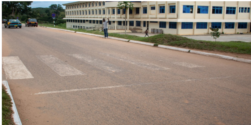
Plate 1: Faded Pedestrian Crossing Site
